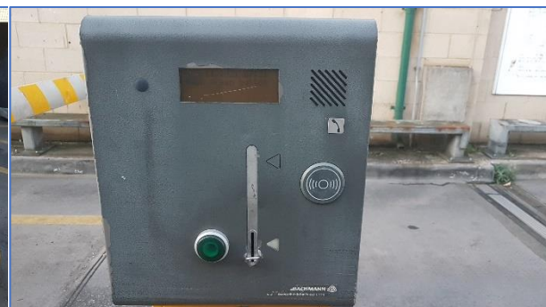
Token operated barrier system (Rock Road)
